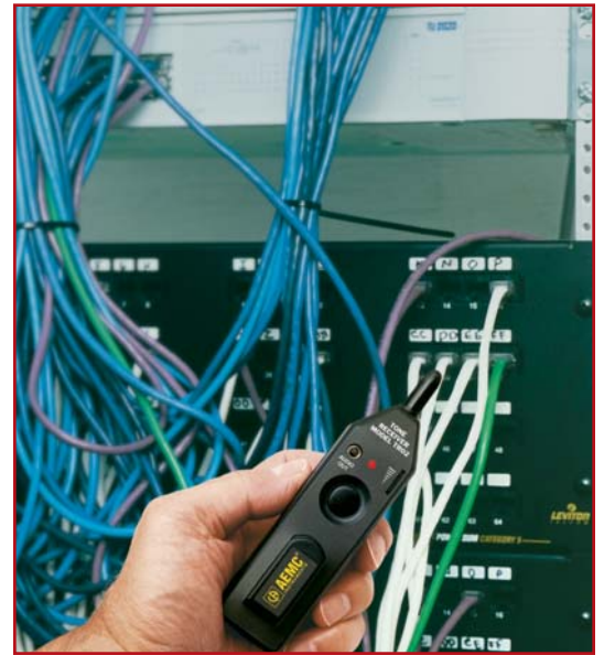
Model TR02 used to find cables in a panel.
